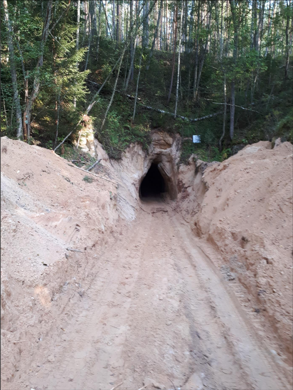
Photo 1. The opened entrance of the cave tunnel through which culvert elements were brought into the section with collapsing risk.
