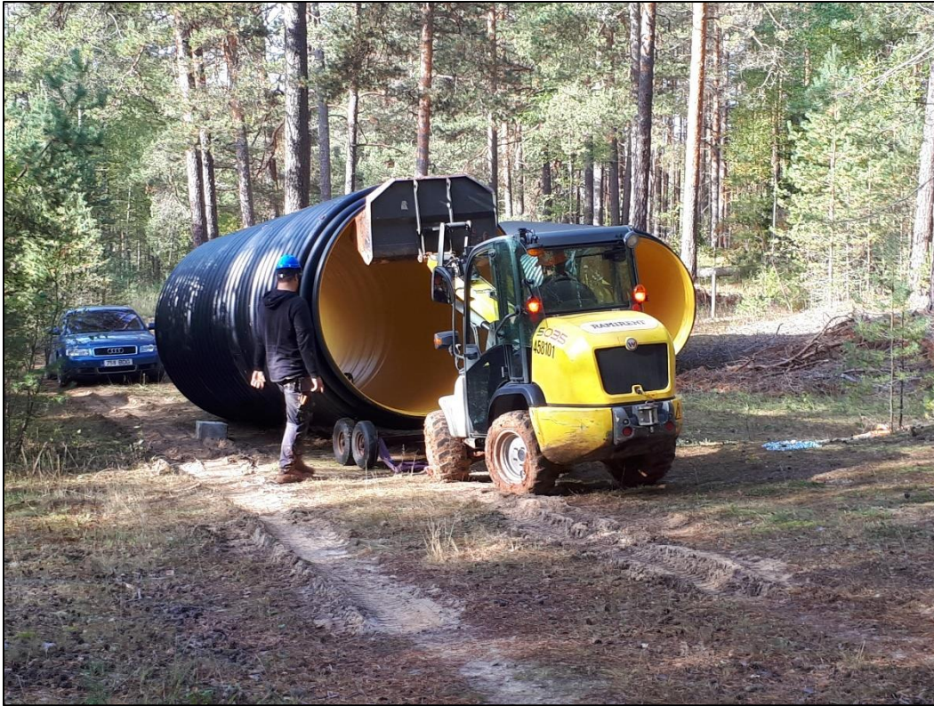
Photo 2. Preparation of pulling-pushing culvert elements with two small size four wheel loadres outside of the cave tunnel.
