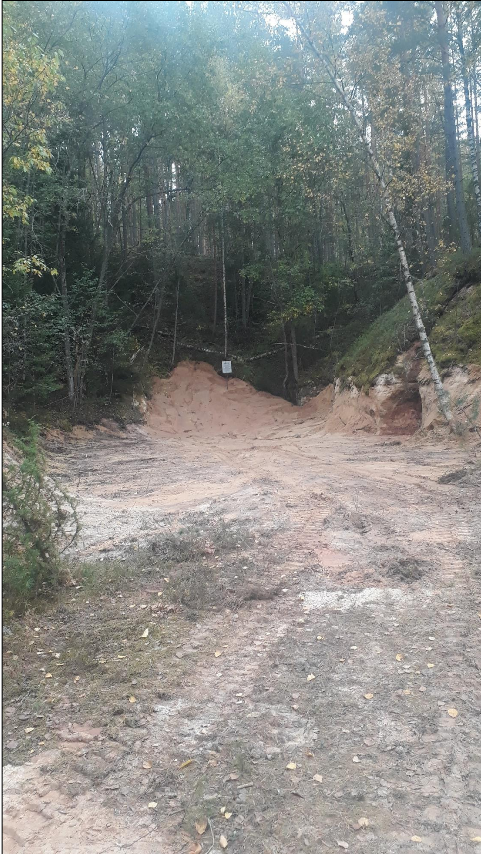
Photo 4. Closed entrance of the cave tunnel after the culvert system was placed.
