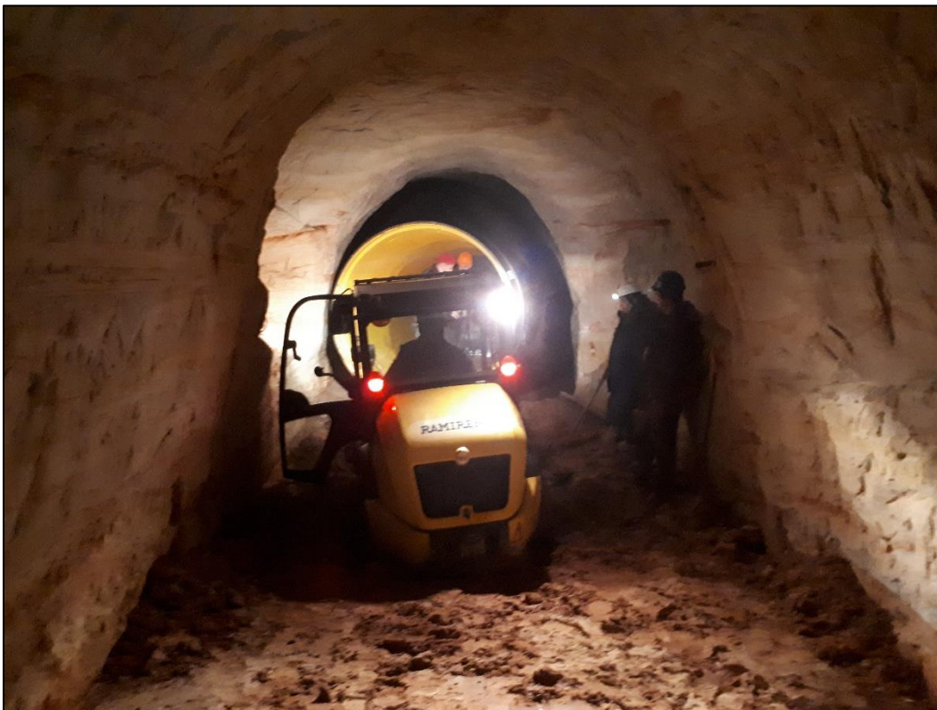
Photo 3. Pulling and pushing culvert elements with two small size four wheel loadres inside of the cave tunnel.
